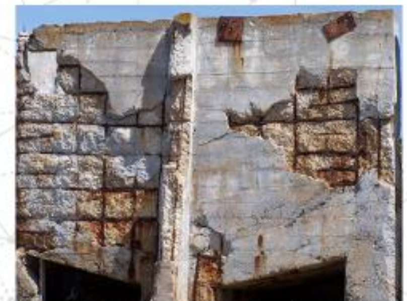
Spalling Due to Corroded Rebar
